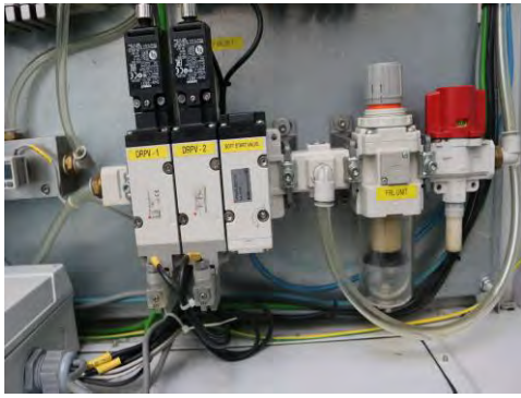
Picture 17 Hazard 2.6, Image 1, Pneumatic Lockable Isolator
