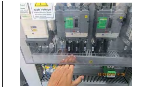
Picture 12 Hazard 2.1, Image 2, Access to live part from Bottom side
