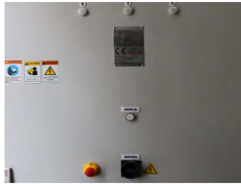
Picture 50 Hazard 5.1, Image 4, Warning signs
