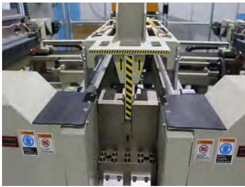
Picture 28 Hazard 3.4, Image 1, Light curtain installed at 342 mm
