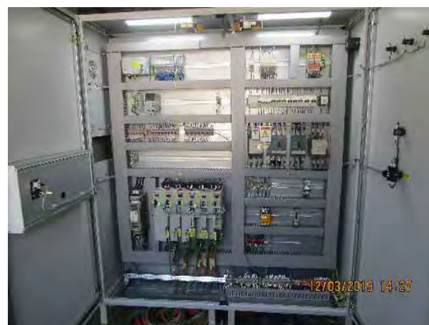
Picture 2 Flex Core Build Machine main control panel
