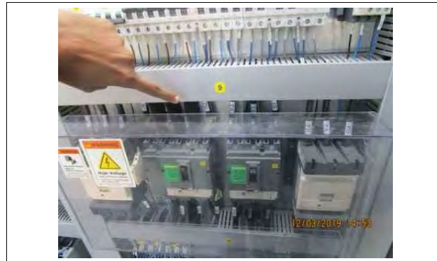
Picture 11 Hazard 2.1, Image 1, Access to live part from Top side
