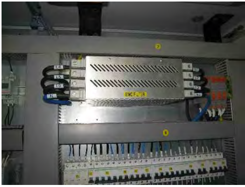
Picture 53 Hazard 5.5, Image 1, EMC Filter
