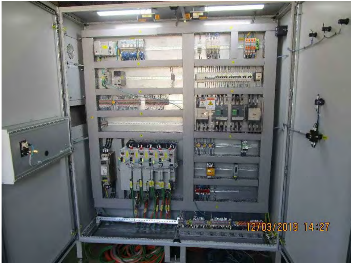
Picture 10 Hazard Related to energy equipment (Electrical & Pneumatic)
