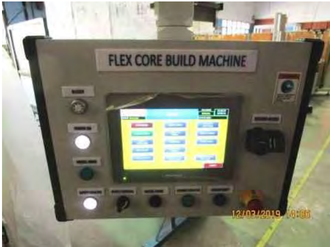
Picture 20 Hazards related to the control system
