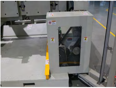
Picture 5 Hazard 1.3, Image 1, Fixed guarding with warning signs
