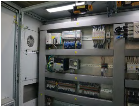
Picture 45 Hazard 4.5, Image 1, Lighting provision in electrical panel
